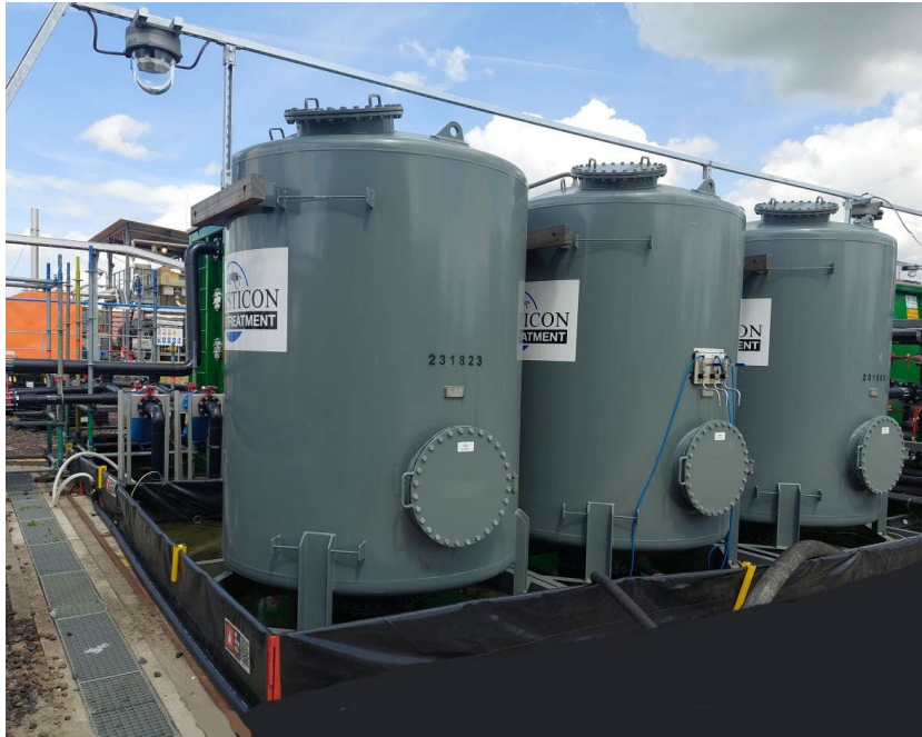
Three-stage ion exchange resin vessel cascade for adsorption of short-chain PFAS at Chemours in Dordrecht, South Holland (Netherlands). Photo: Chemours Dordrecht, courtesy of Logisticon Water Treatment
