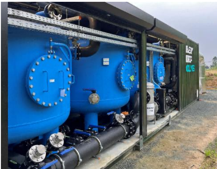
Mobile, modular system for PFAS removal from water. The Lewatit TP 108 DW ion exchange resin from LANXESS is used for filtering.
