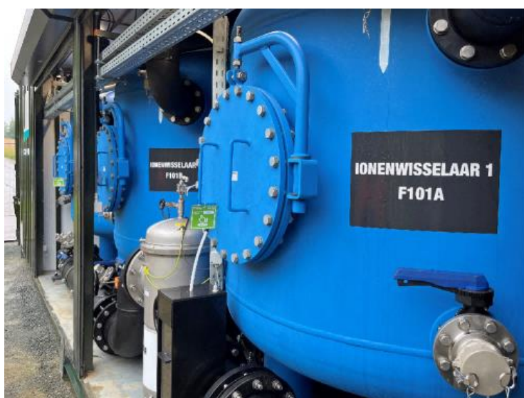
Mobile, modular system for PFAS removal from water. The Lewatit TP 108 DW ion exchange resin from LANXESS is used for filtering. Photos: De Watergroep
