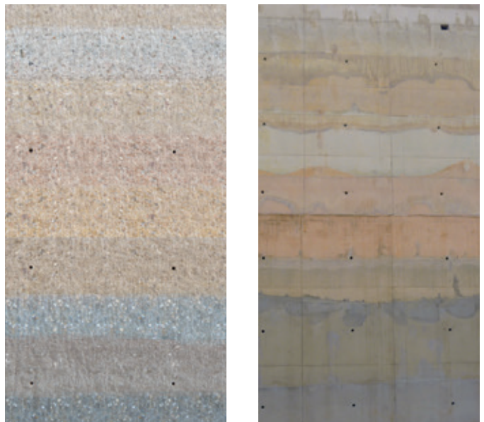
■ Sample walls to test the color development before and after the grinding of the surface.
