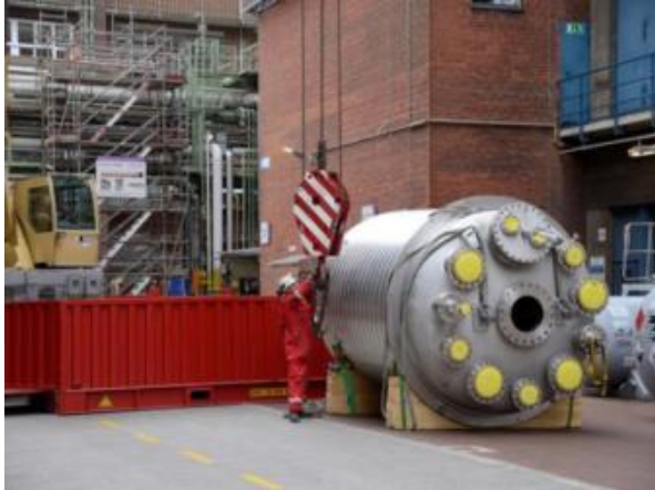
A crane lifts an 11-metric-ton stirrer vessel to its place on floor 3 of the building and positions it with great precision. Photo: Saltigo GmbH
