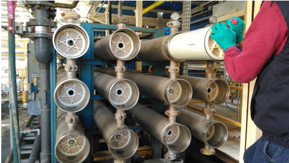
Pressure vessels in a reverse osmosis unit in Turkey are loaded with Lewabran RO membrane elements from LANXESS. Photo: Burkut
